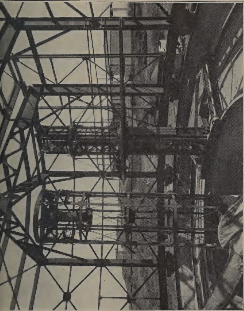
FIGURE 4. The 60-inch reflector on Harvard Kopje, and the steel framework of the turret under construction. To the right of the telescope is the electrically driven observing platform, which moves on a circular track.
